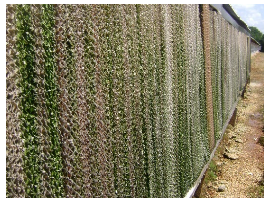
Figure 14. Algae growth on damaged pads
