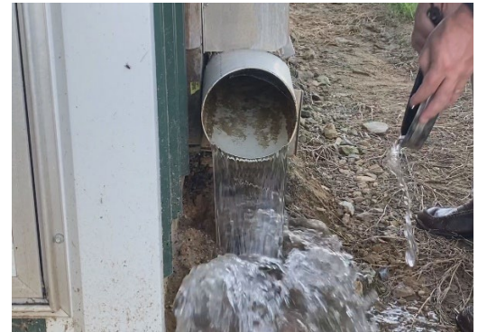
Figure 13. Dumping pad system reservoir
