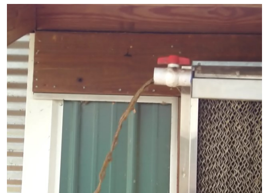
Figure 18. Flushing water distribution pipe
