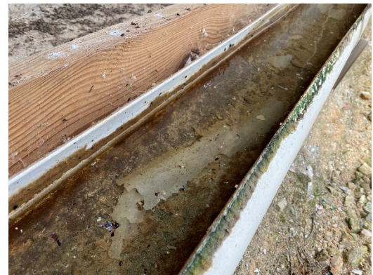
Figure 10. Dirt and mineral build-up in pad system reservoir
