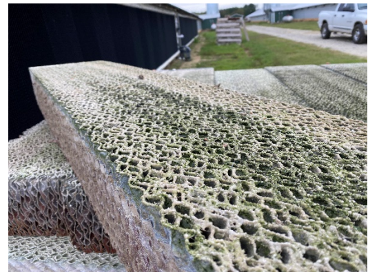
Figure 17. Pads replaced due to excessive mineral build up
