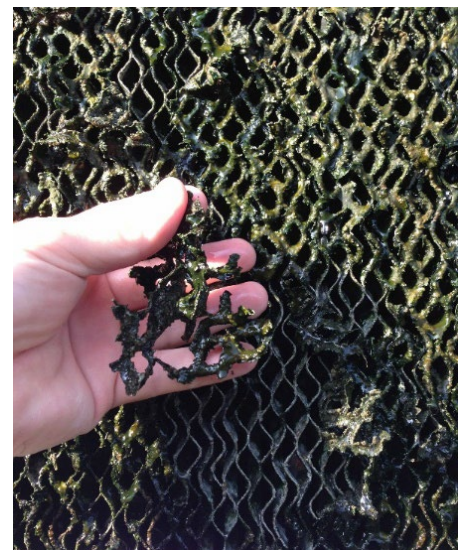
Figure 16. Severe algae growth
