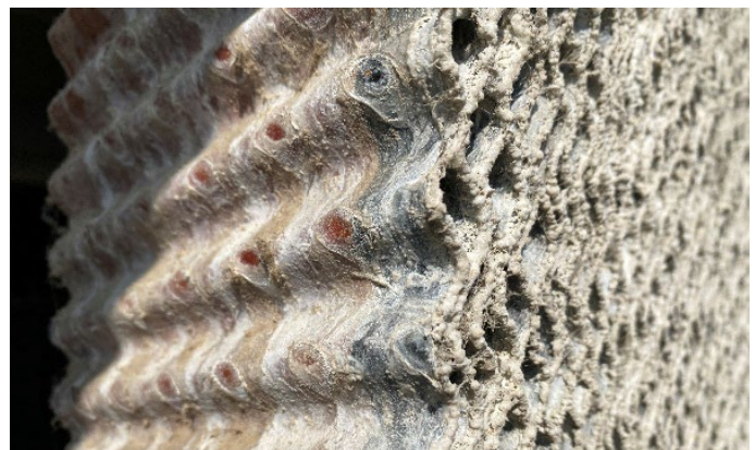
Figure 12. Mineral build-up on exterior and interior pad surfaces
